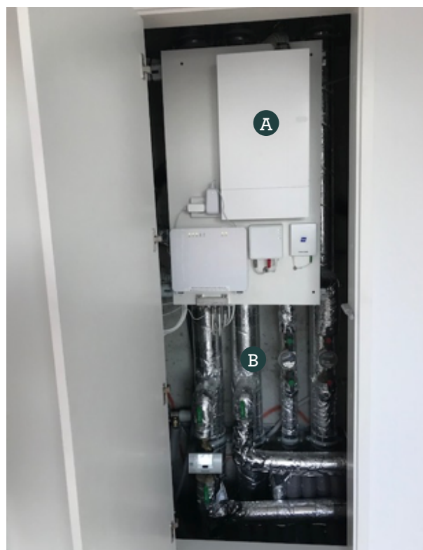
A — Electrical installations
