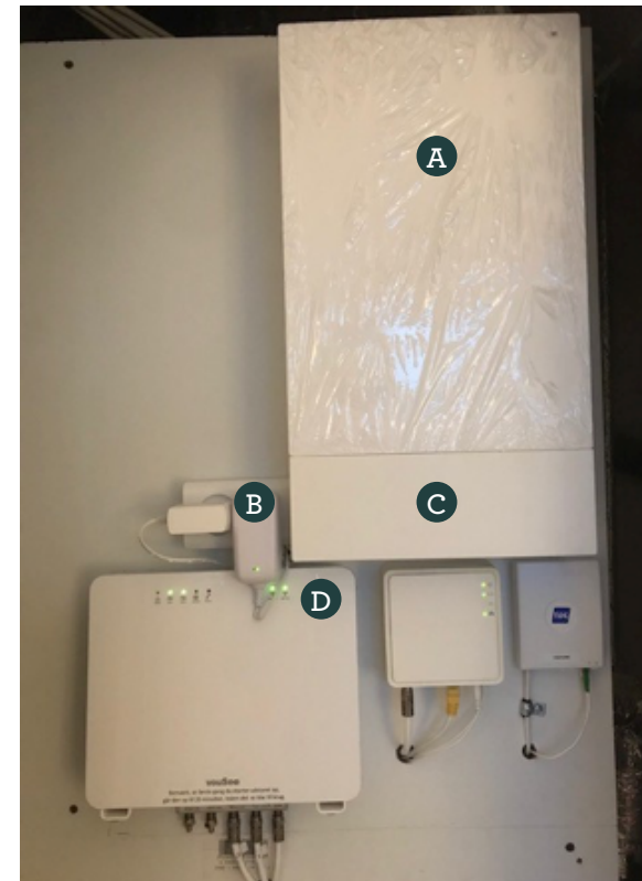
A — Electrical panel
