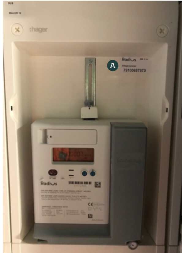
A - Unit number: The unit number and address are placed in the flat's electrical box.
