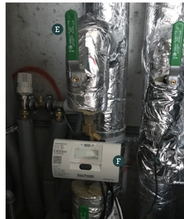
E — District heating: Shut-off valve for district heating. Do not adjust the district heating controls.
