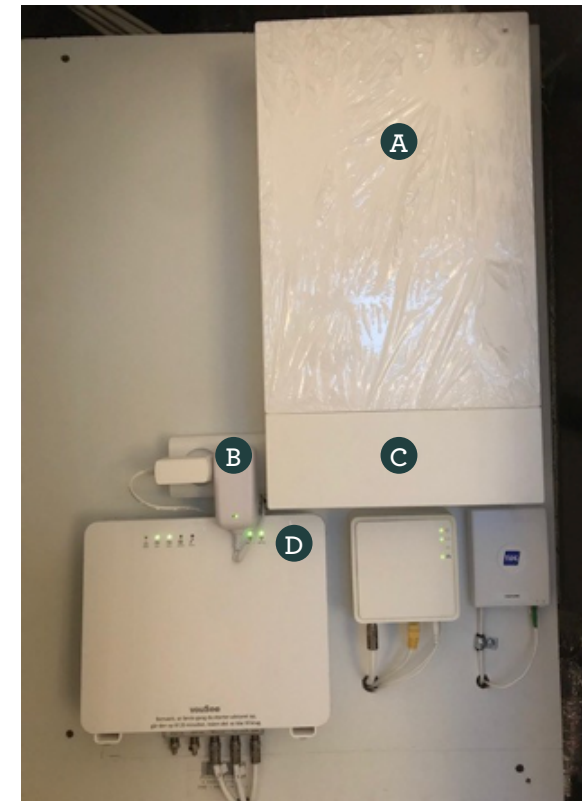
A – Electrical panel B – Cable TV / antenna box C – Fibre network box D – Router
