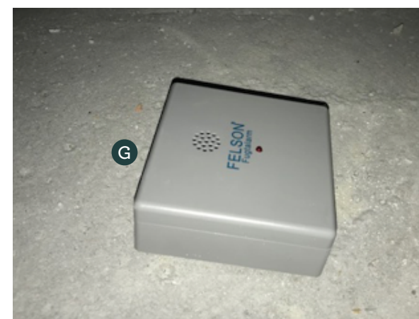
G — Moisture alarm: At the bottom of the technical shaft, a moisture alarm is installed. This alarm is designed to alert you to leaks in the shaft with a loud, high-pitched tone.
